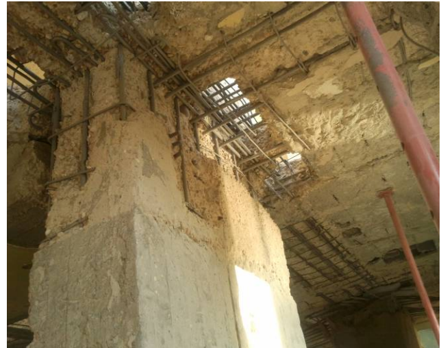
Fig. (1) Bad quality concrete at upper part of column
