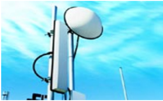
Figure1.2 WiMAX transmitting tower
